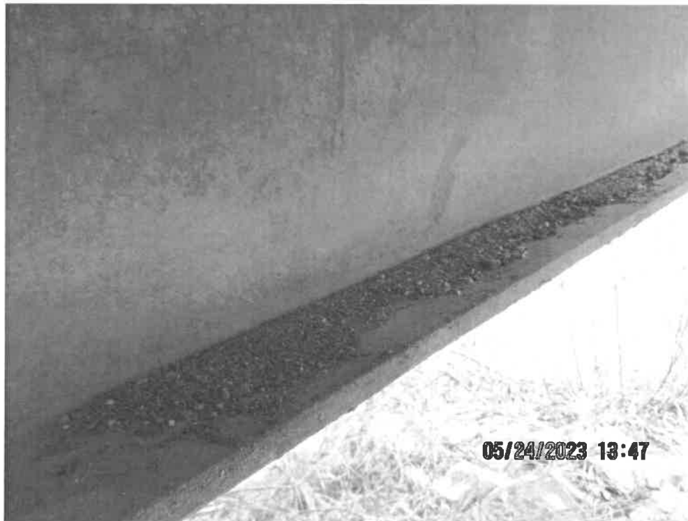
Photo 17: Gravel accumulation at stringer.
