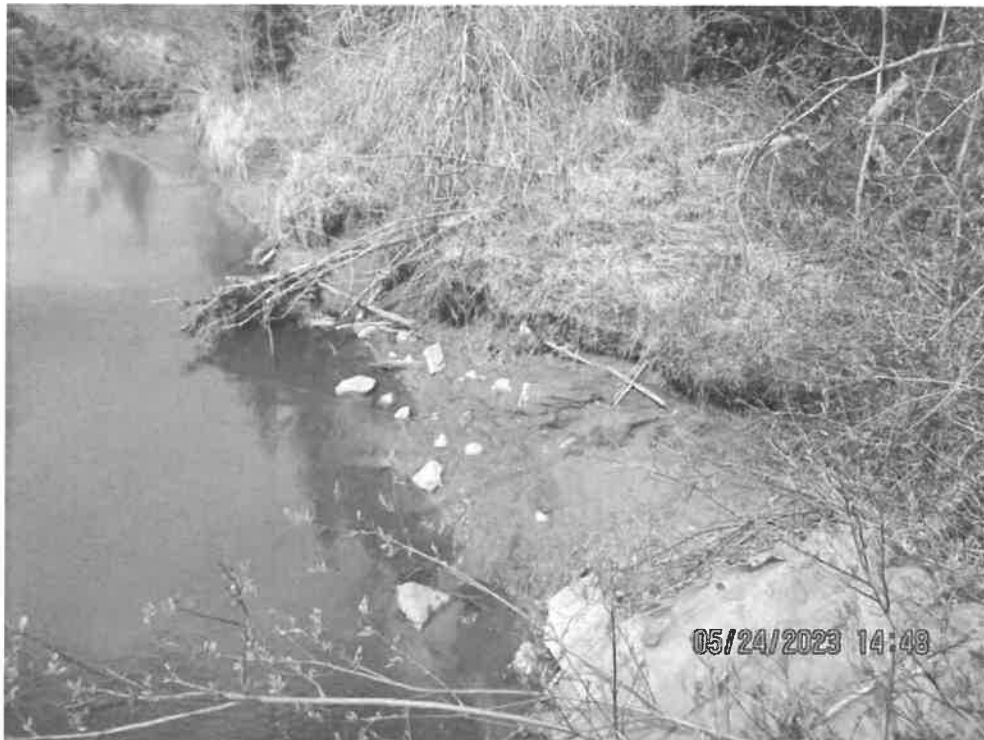
Photo 8: Erosion at embankment.
