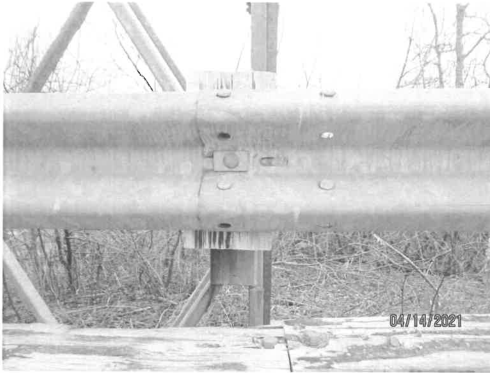
Photo 19: Missing bolts at guide rail (typ.).
