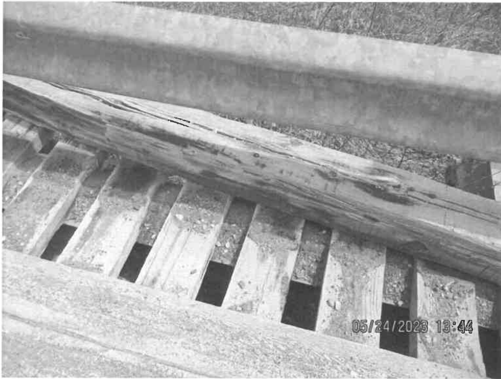
Photo 15: Impact damage at northeast curb.
