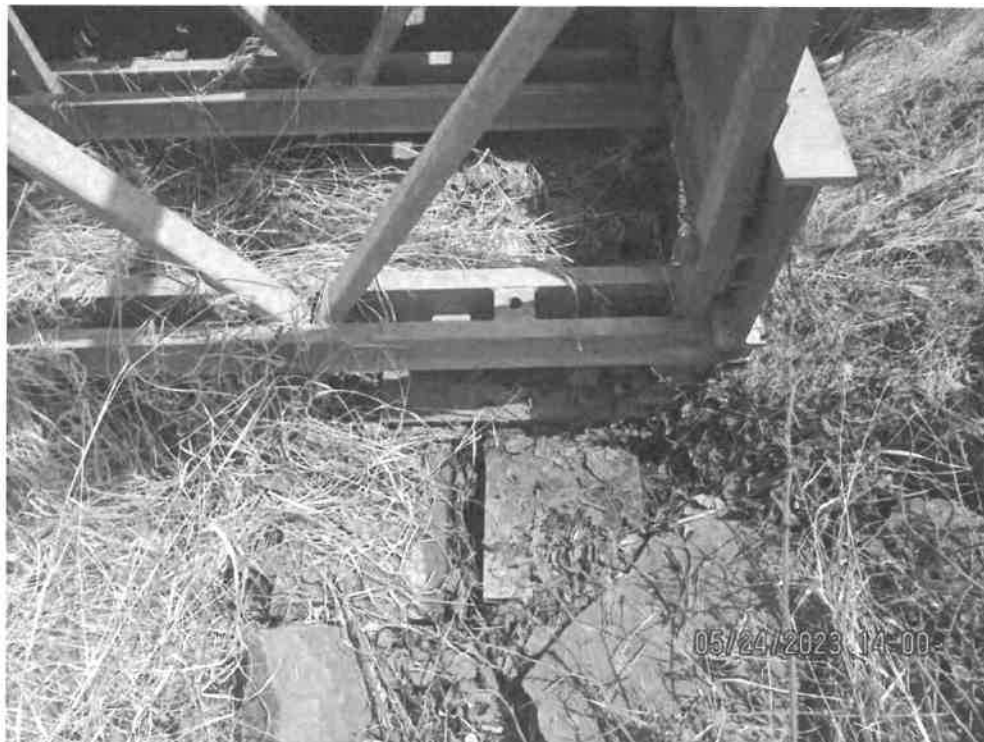
Photo 24: Separated bearing timbers at south abutment.
