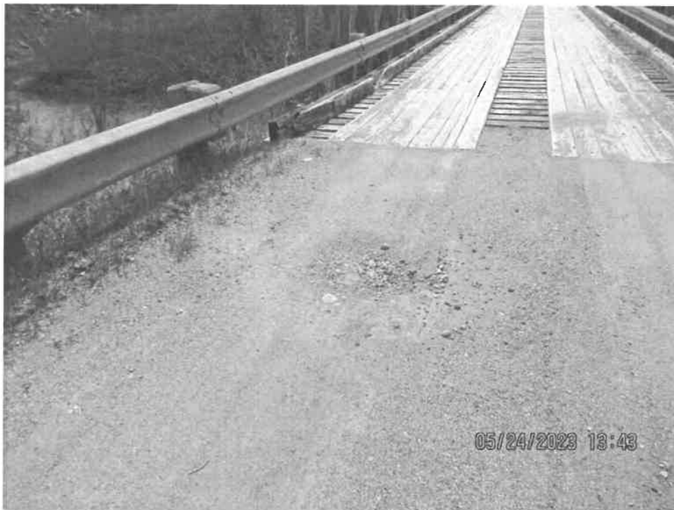
Photo 20: Severe potholes at north approach.
