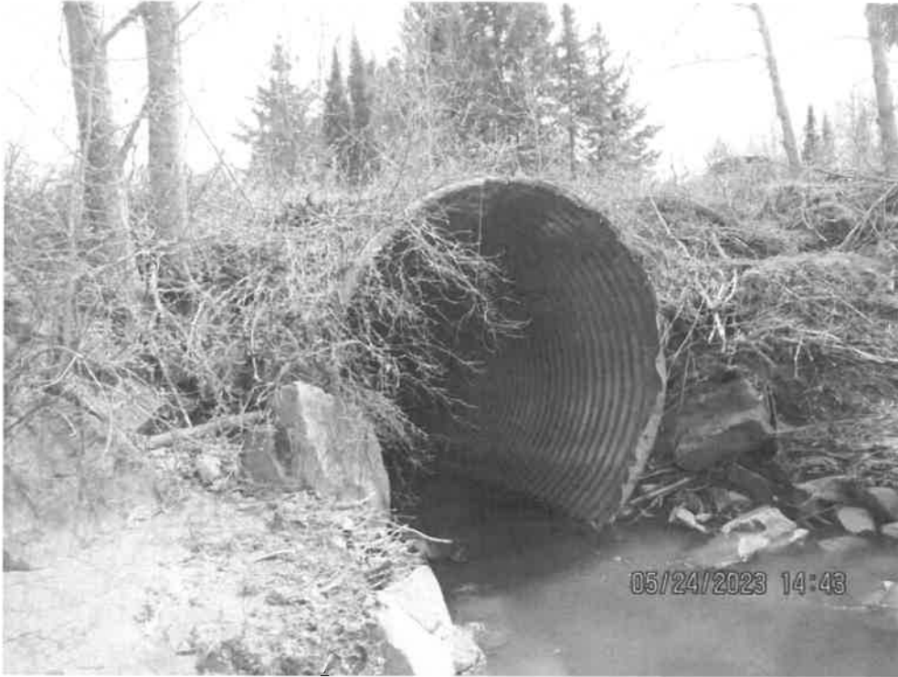
Photo 3: North end (inlet) of culvert with edge damage and stream debris.
