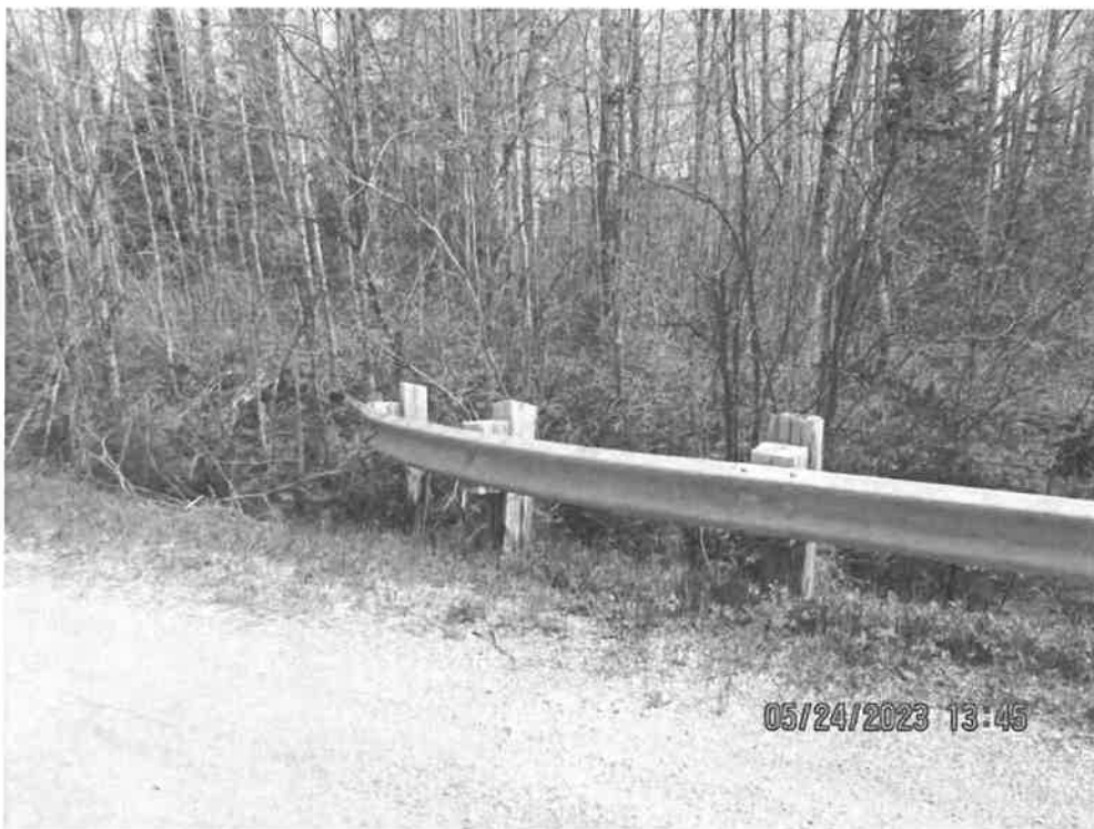
Photo 18: Improper guide rail end termination (typ.).
