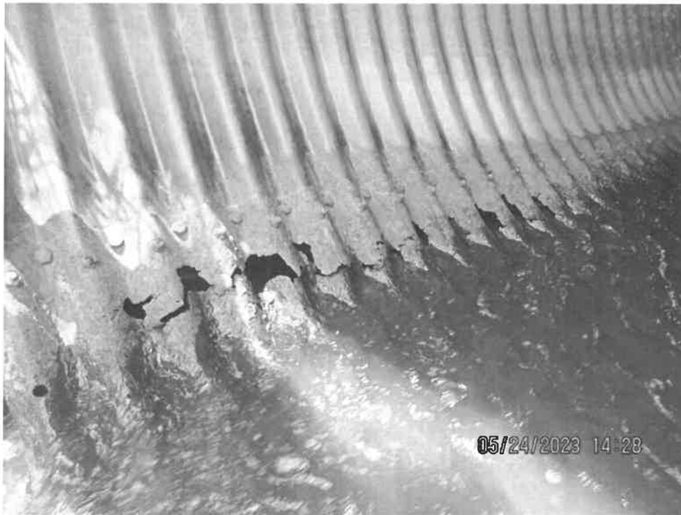
Photo 10: Perforations in culvert (typ.).
