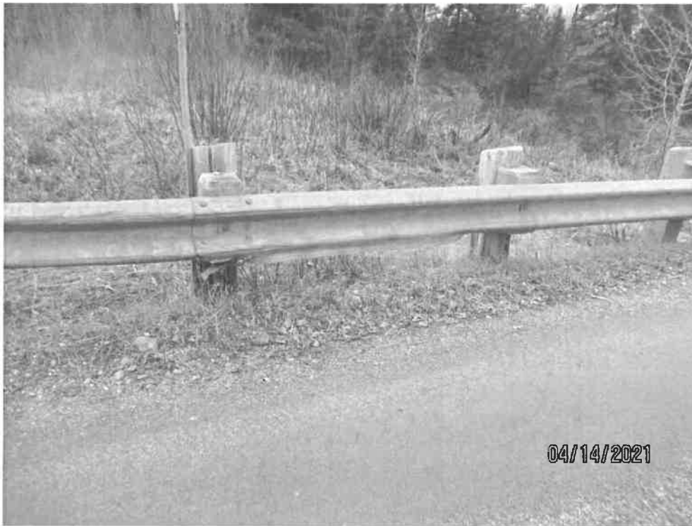
Photo 13: Impact damage at southwest guide rail.
