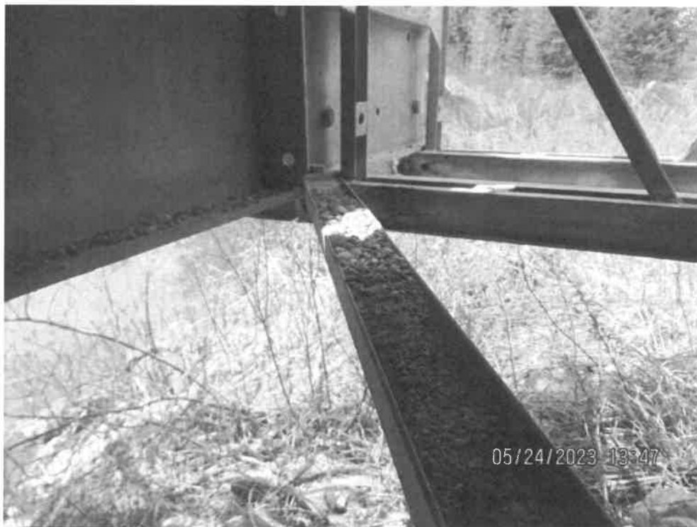
Photo 16: Gravel accumulation at sway bracing.
