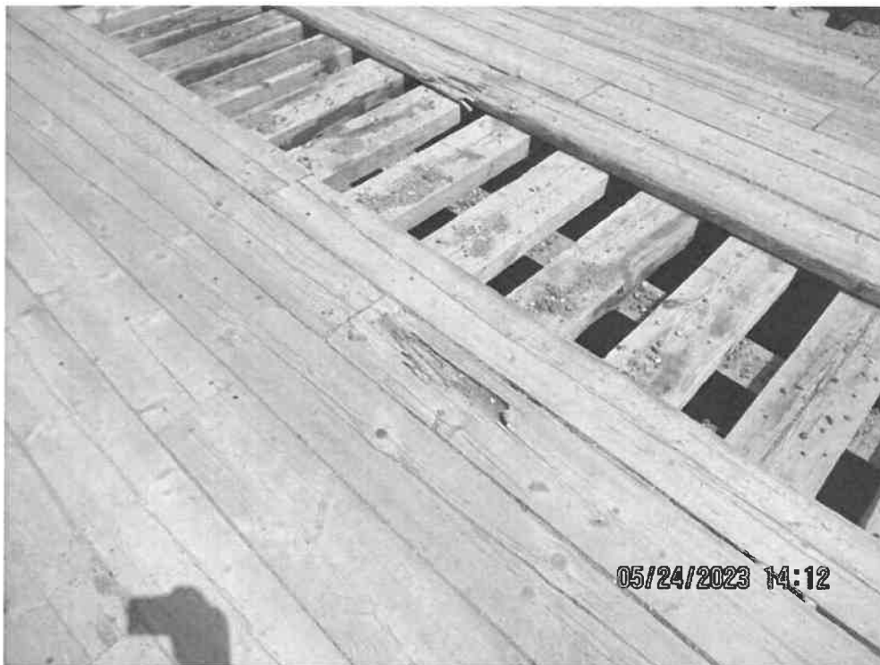
Photo 14: Severely rotten wearing surface plank.
