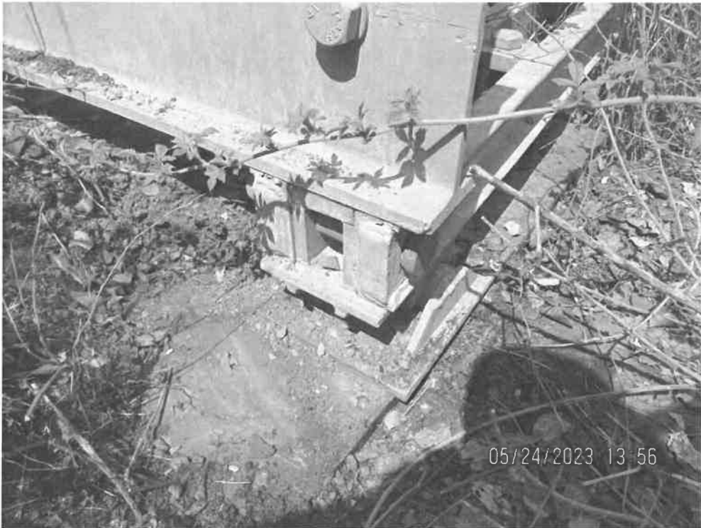
Photo 25: Base plate shifted off centre of bearing plate.
