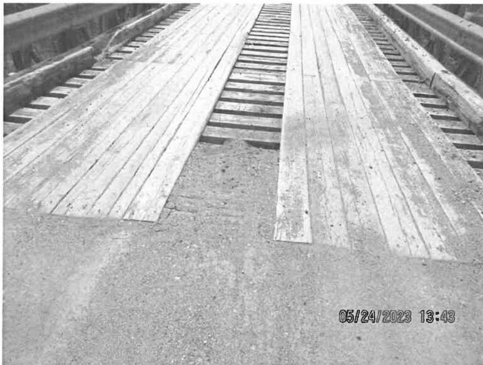
Photo 22: Gravel accumulation at approach span (typ.).
