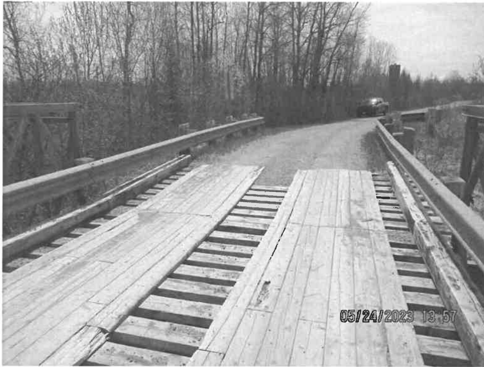
Photo 23: Significant change in centerline profile at south approach span.
