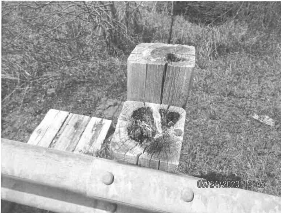
Photo 21: Medium end rot at post and offset.
