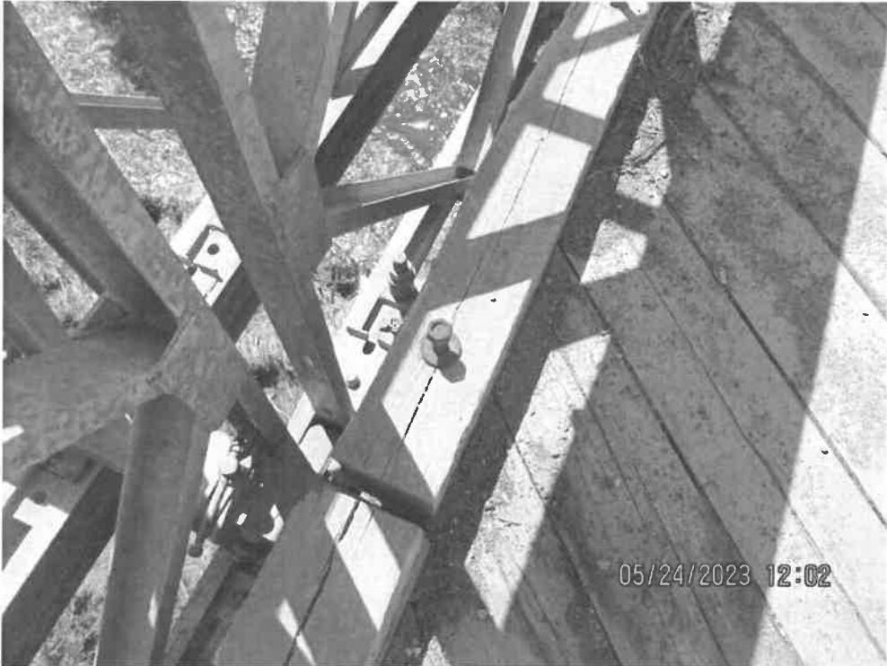
Photo 15: Loose/missing bolt at curb (typ.).
