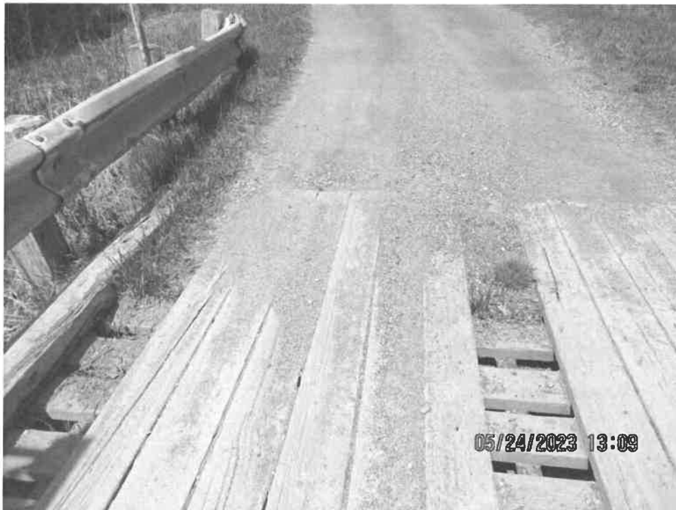
Photo 26: Gravel accumulation at approach (typ.).
