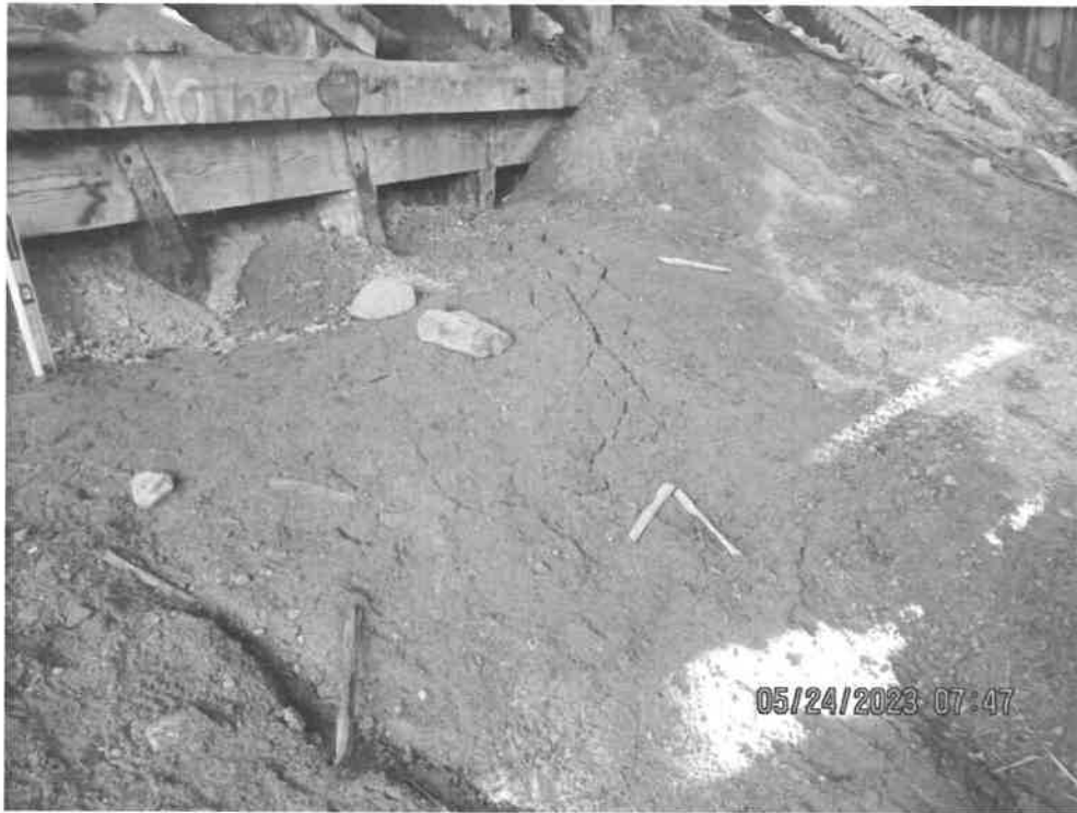
Photo 43: Cracks in soil between Bent #12 and #13.
