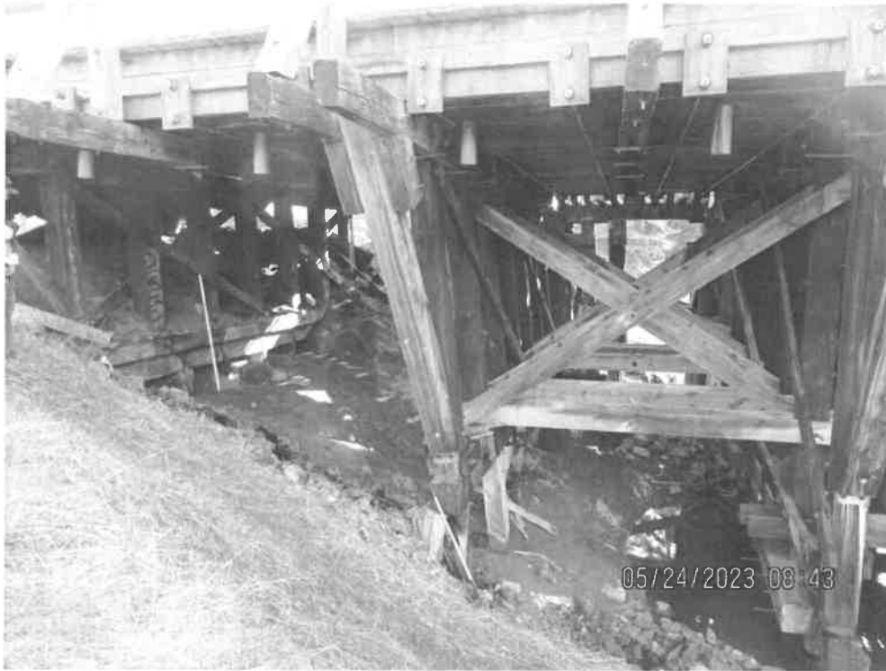
Photo 39: Rotation of piles and pile cap at Bent #12.
