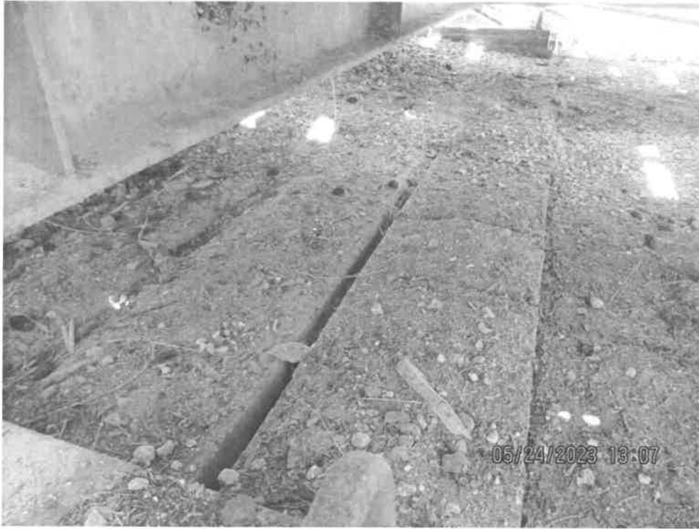
Photo 23: Gravel accumulation at abutment (typ.).
