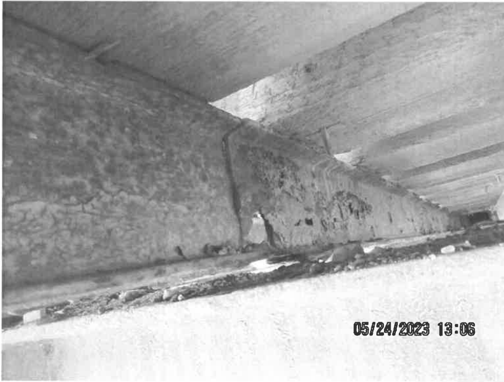
Photo 21: Stringer set not bearing on transom.
