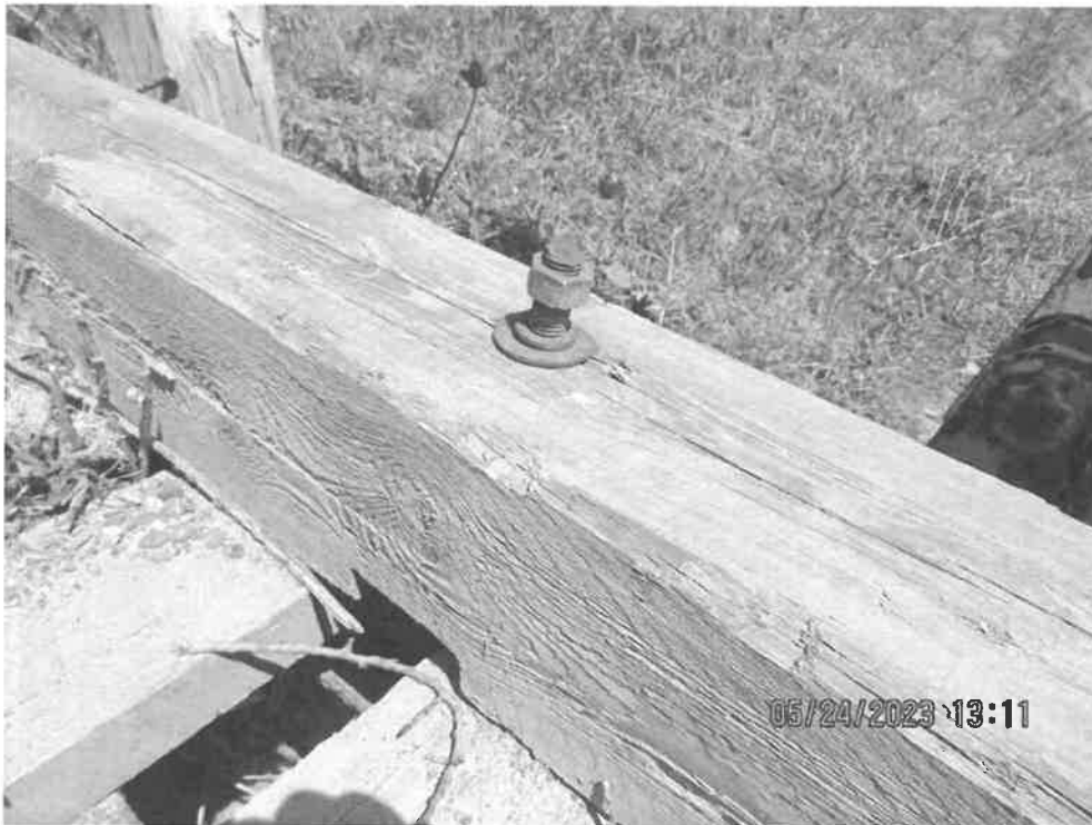
Photo 16: Loose bolt at curb (typ.).
