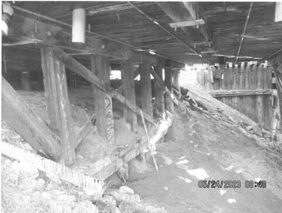
Photo 34: Severe erosion at north embankment.
