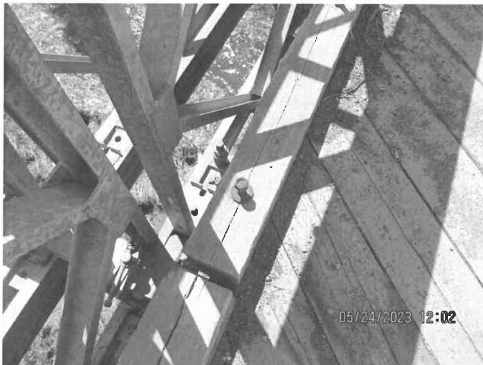
Photo 24: Loose curb bolts (typ.).
