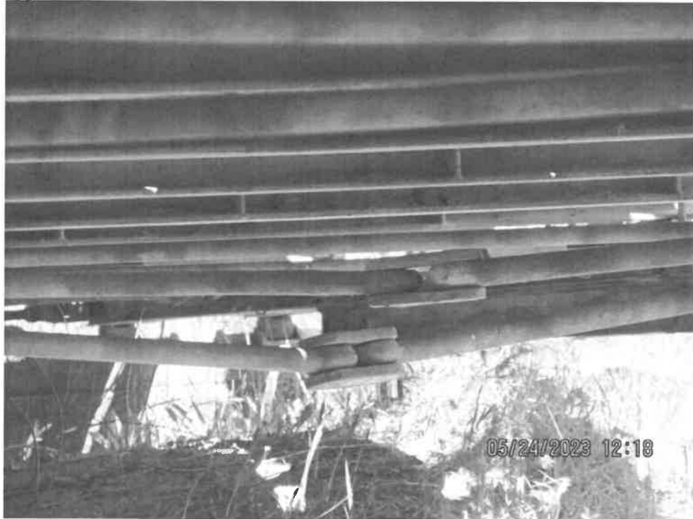
Photo 22: Loose sway bracing beneath bridge.
