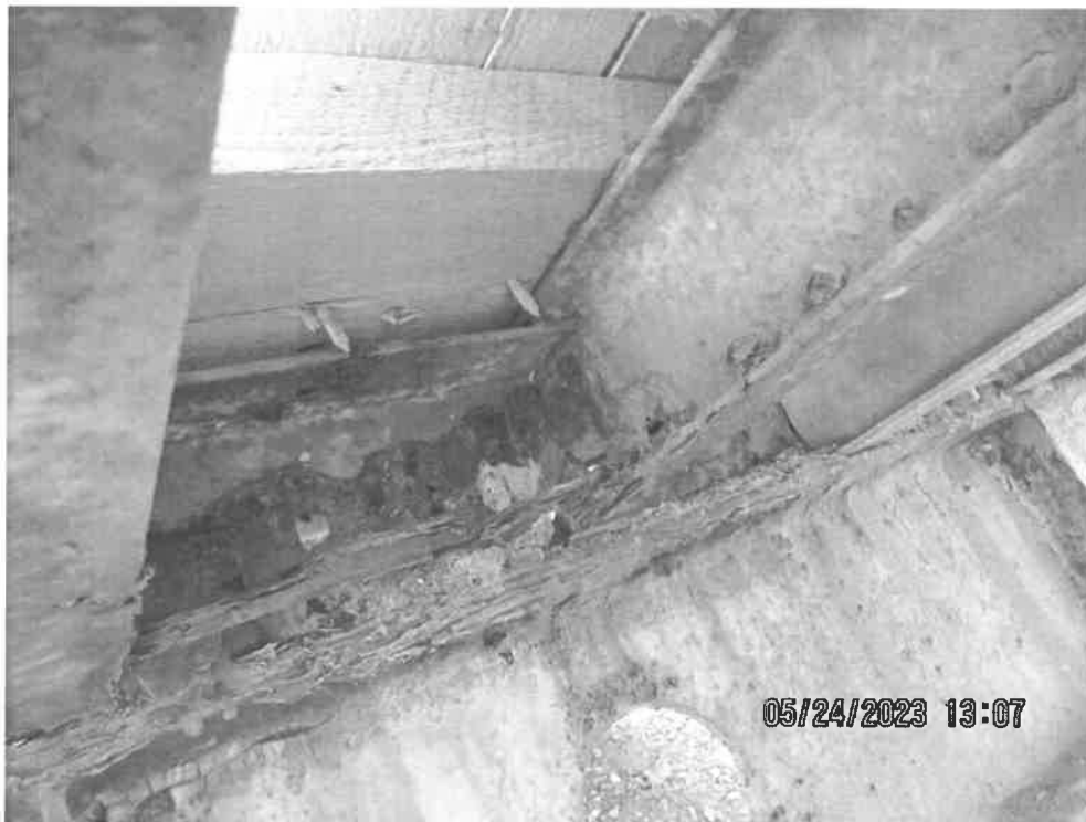
Photo 22: Severe corrosion at end diaphragm of stringer set.
