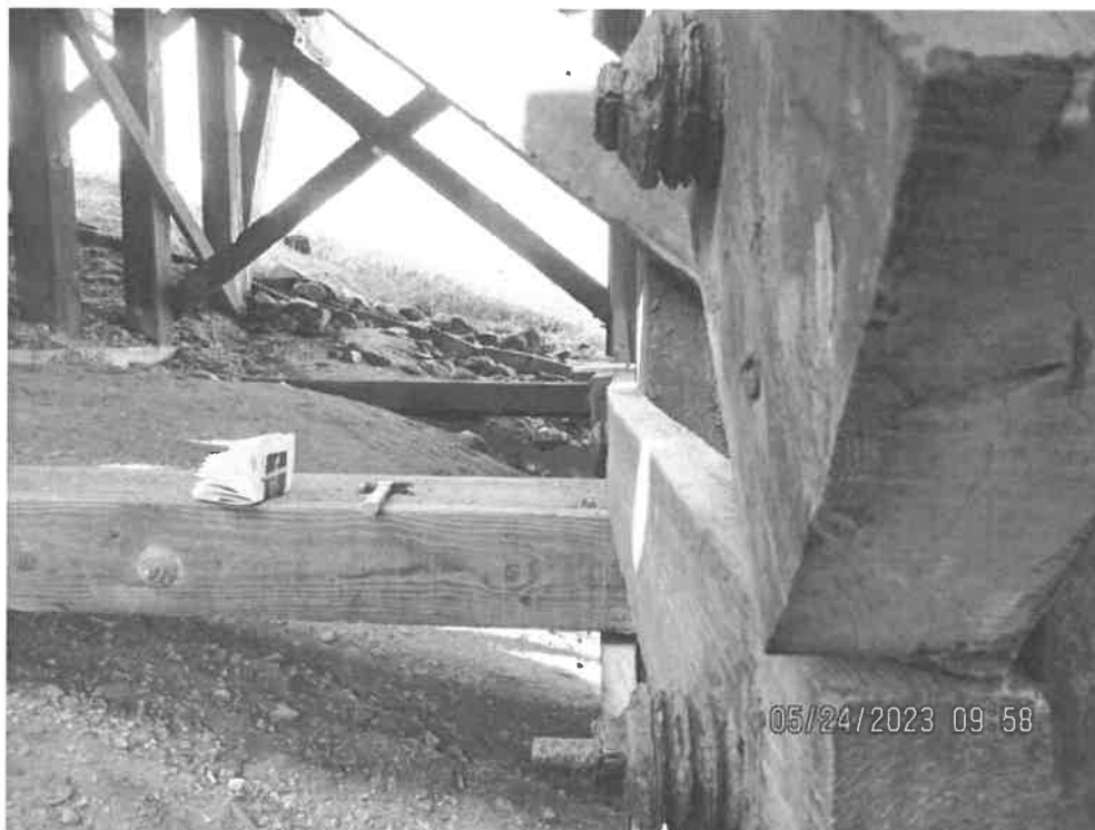
Photo 46: Typical translation of piles and bents.
