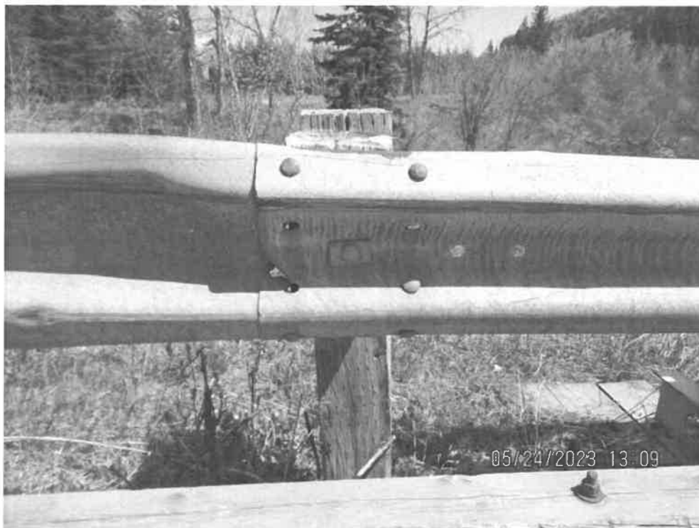
Photo 18: Missing bolts at guide rail splice (typ.).
