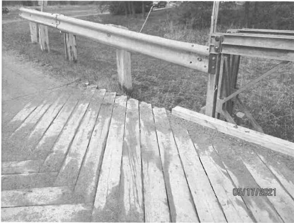
Photo 21: Impact damage at guide rail. Missing curb at 4 corners of approaches.
