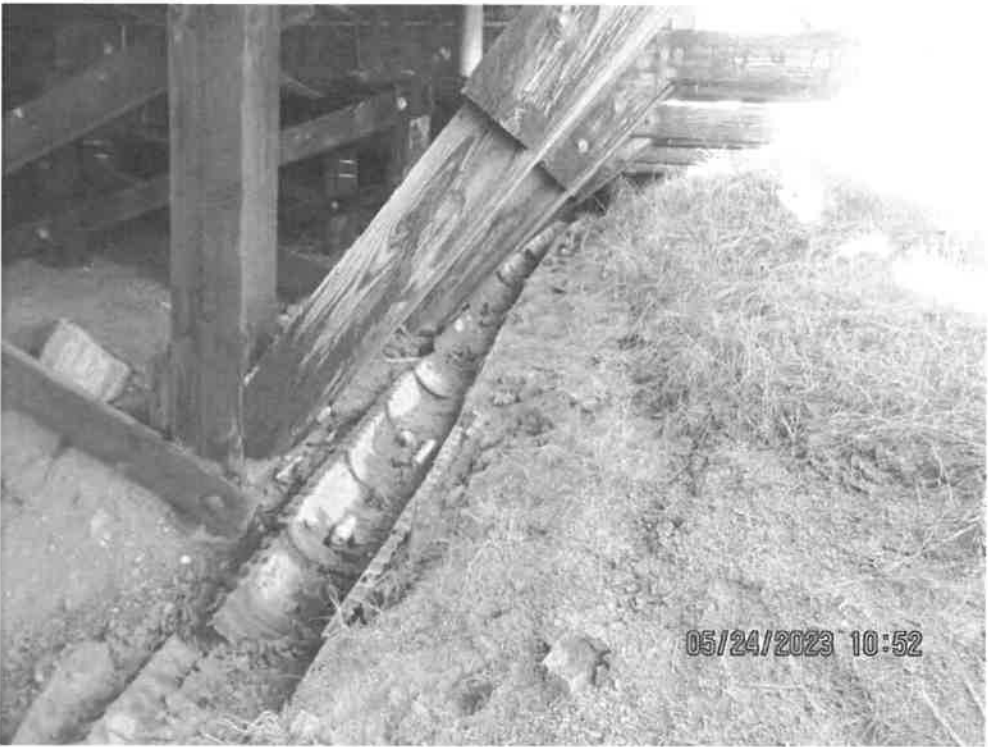
Photo 32: Severe corrosion at drainage culvert at southwest corner.
