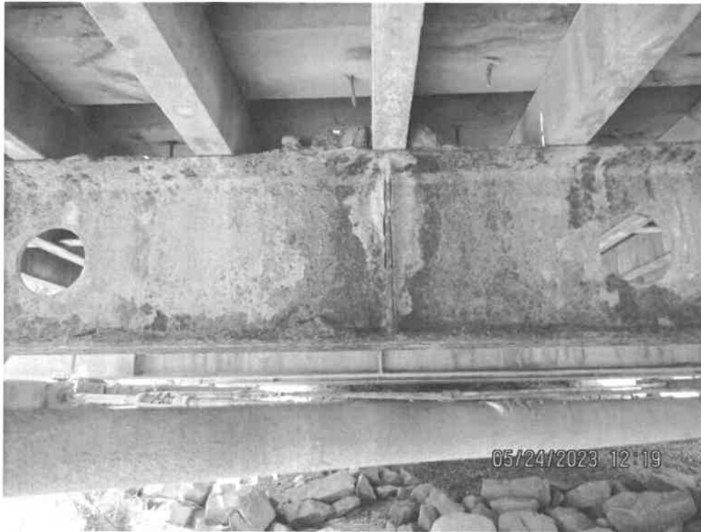
Photo 23: Medium corrosion at transom.
