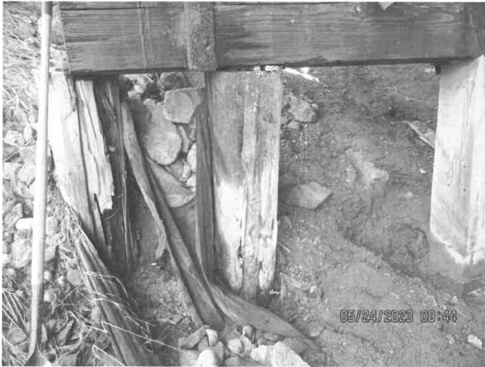
Photo 27: Very severe rot at 8 th pile from east at Bent #12.
