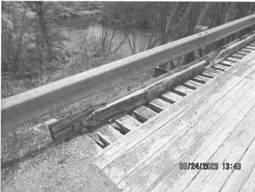
Photo 24: Severe impact damage at curb.
