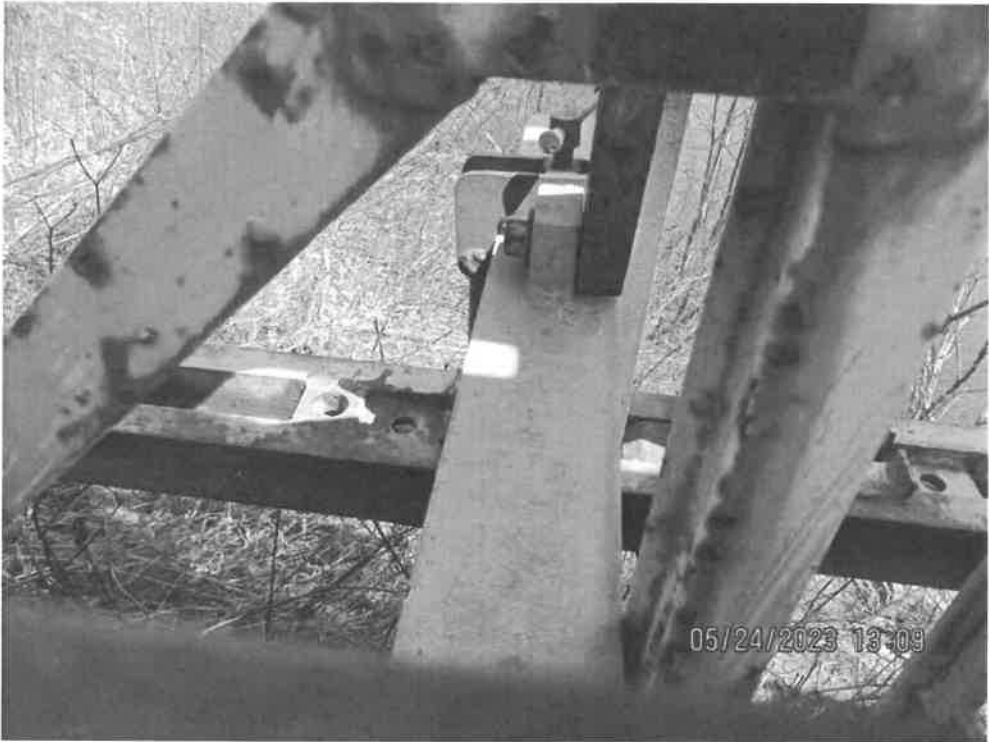
Photo 19: Missing transom clamp at east side.
