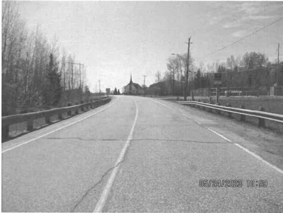
Photo 17: Medium longitudinal crack at south approach.
