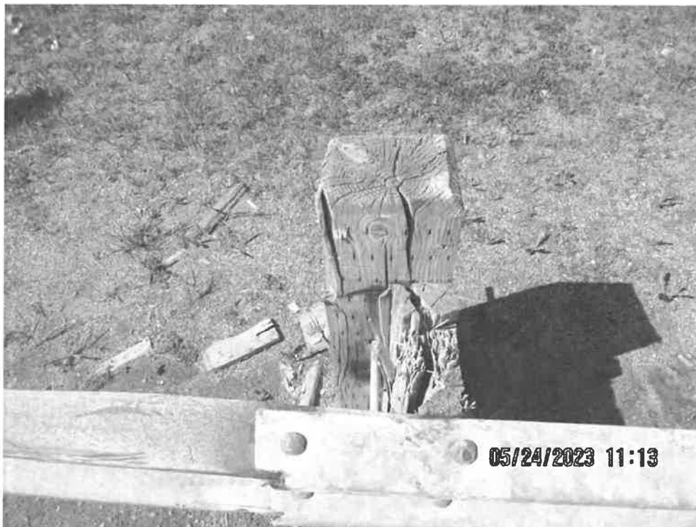
Photo 20: Severe rot at offset at northeast approach.
