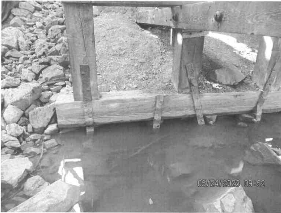
Photo 37: Strapping buckled at pile (typ.).
