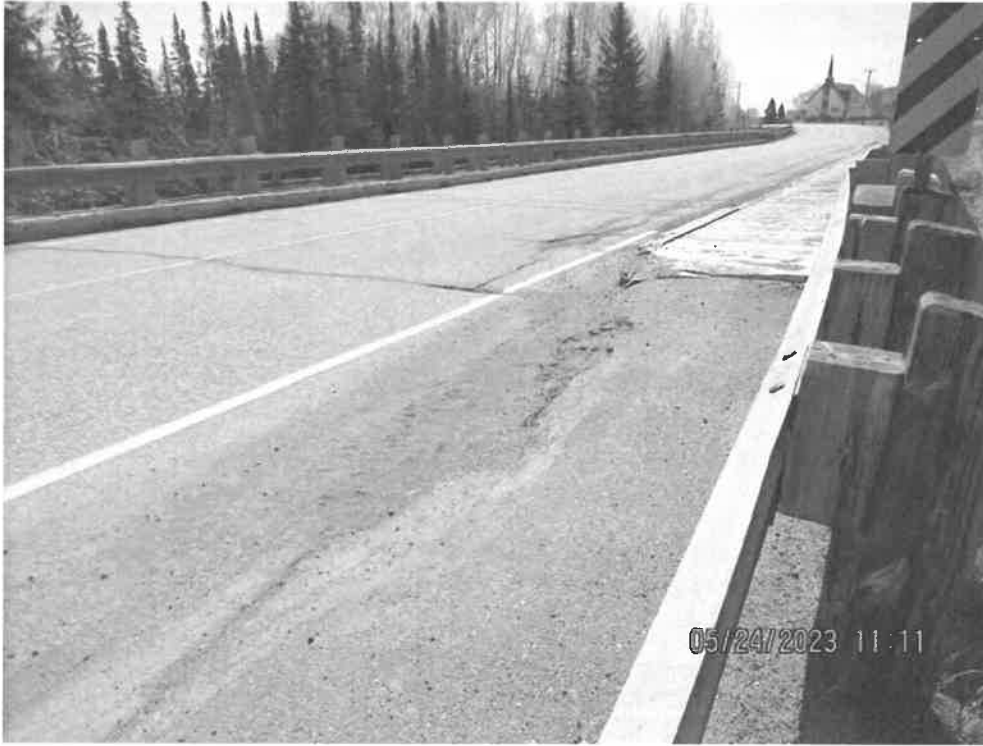
Photo 15: Impact damage at asphalt at north walkway approach.
