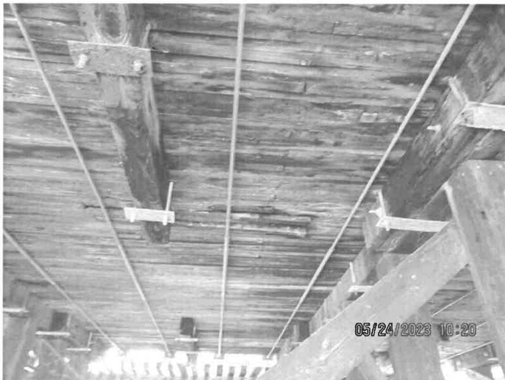
Photo 30: Severe separation of deck timbers (typ.).
