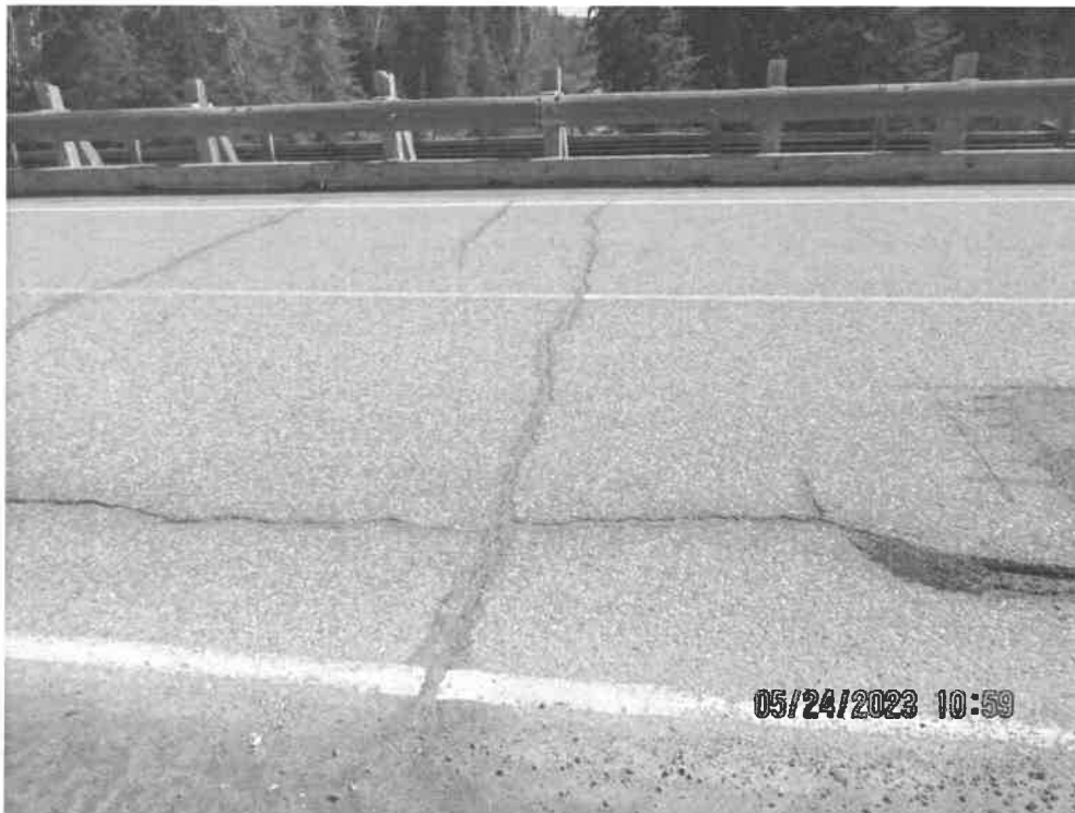
Photo 16: Severe transverse crack at asphalt wear surface (typ.).
