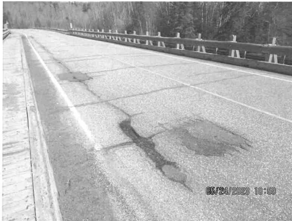
Photo 24: Severe longitudinal crack full length of deck at southbound lane.
