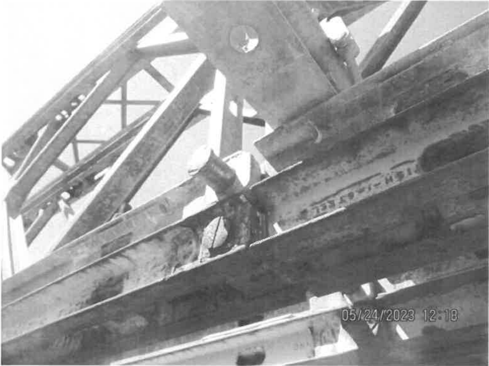
Photo 17: Loose panel pin.
