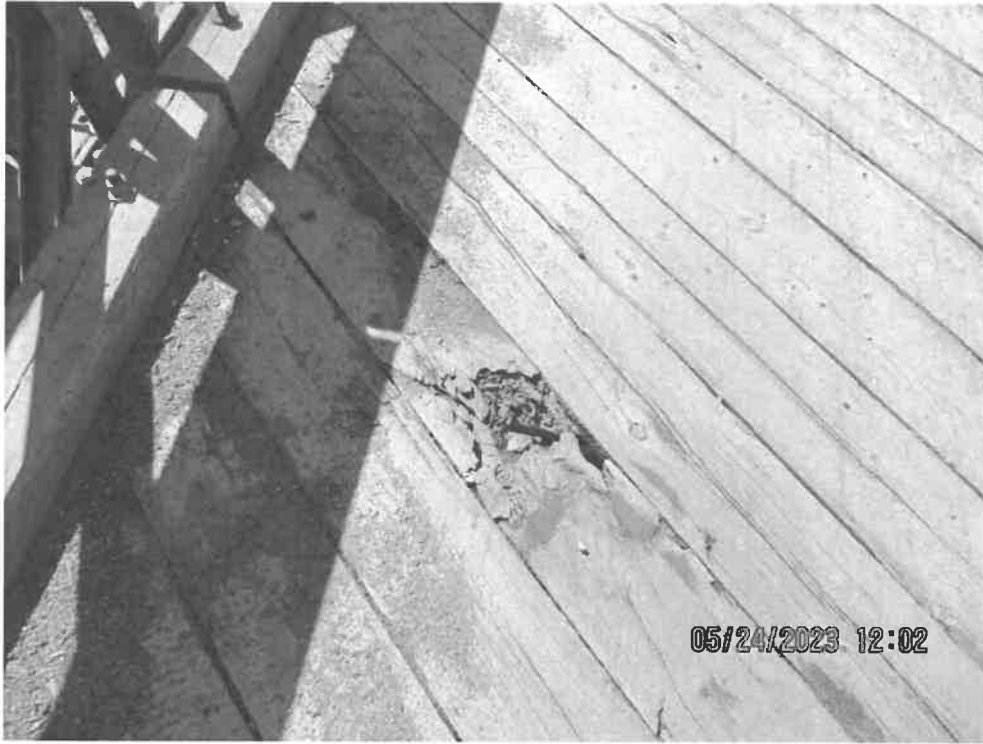
Photo 25: Severe rot at wearing surface.
