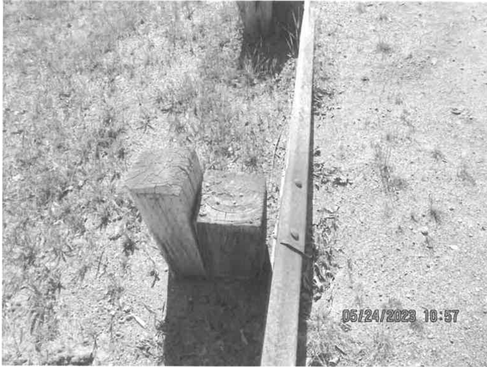
Photo 21: Missing bolt at guide rail to post connection.
