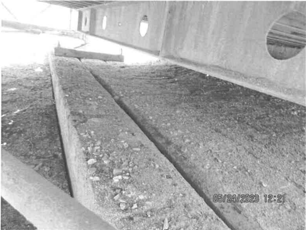
Photo 27: Gravel accumulation at bearing timber (typ.).
