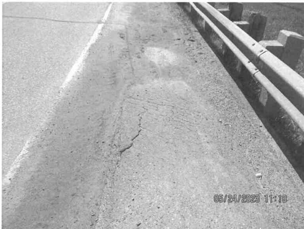
Photo 18: Medium cracking at pedestrian walkway.
