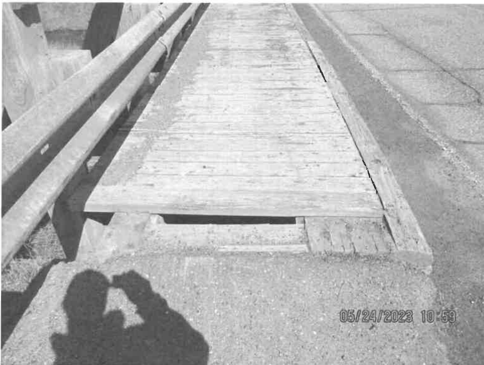
Photo 22: Three missing deck timbers at walkway.
