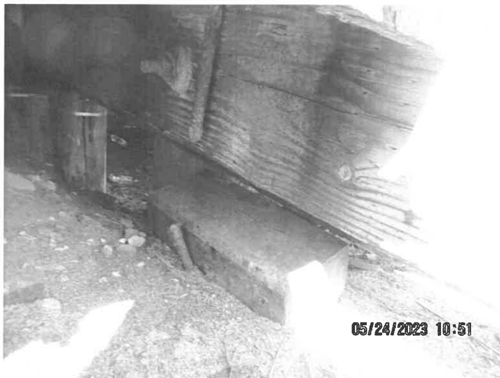
Photo 36: Broken thru-bolt at clamp at Bent #2.
