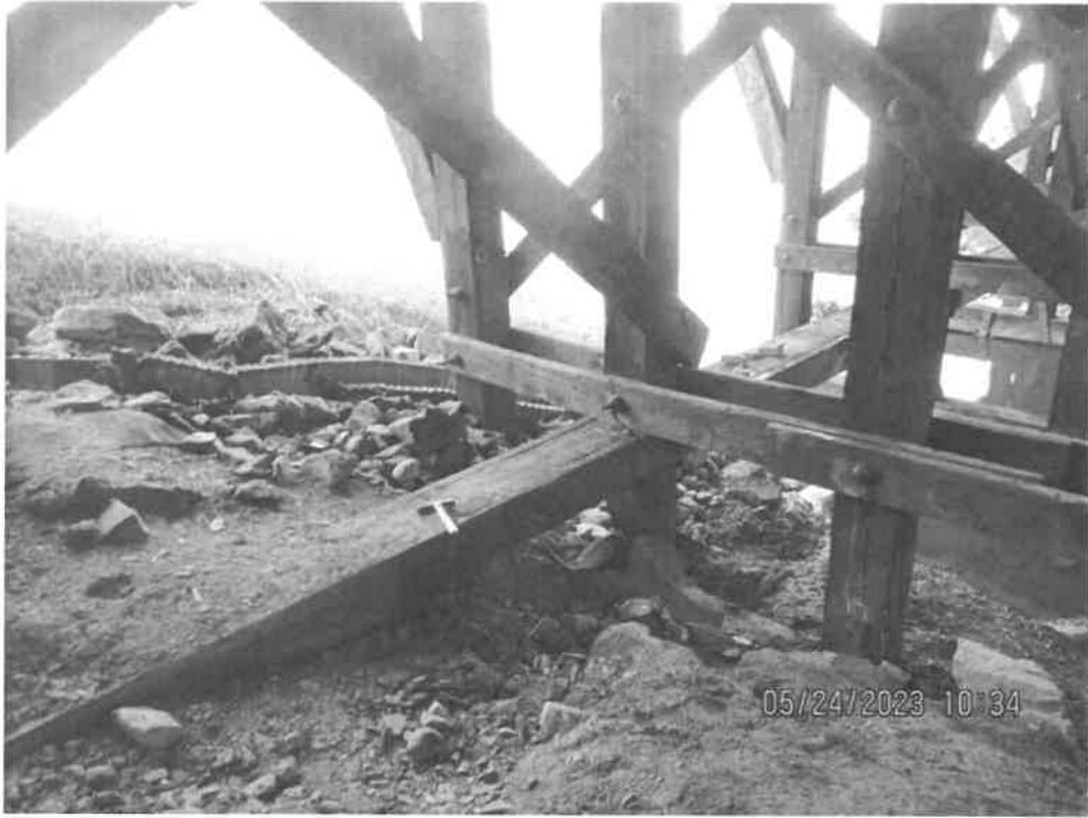
Photo 33: Severe erosion at south embankment.
