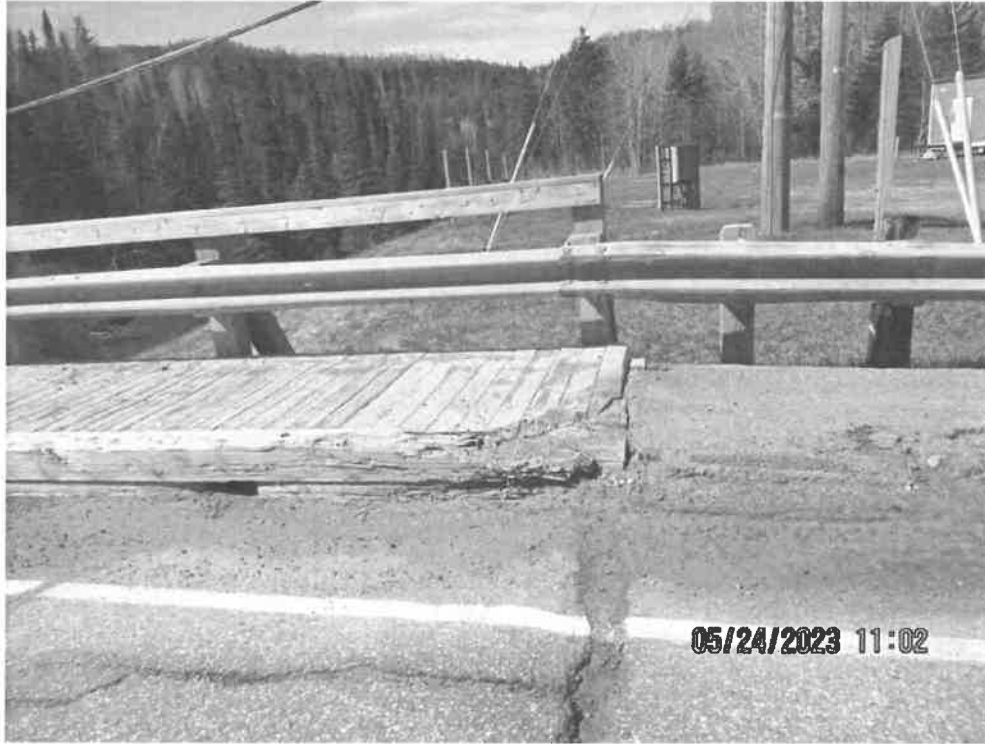
Photo 23: Impact damage at curb at north end.
