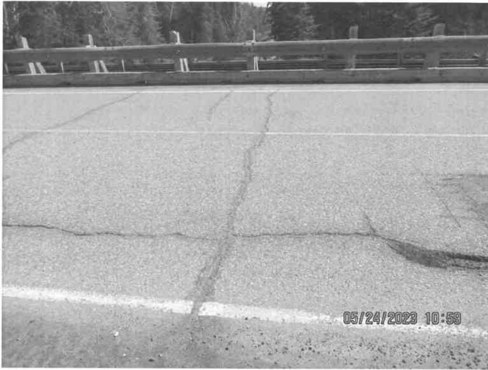
Photo 25: Severe transverse cracks full width of deck.
