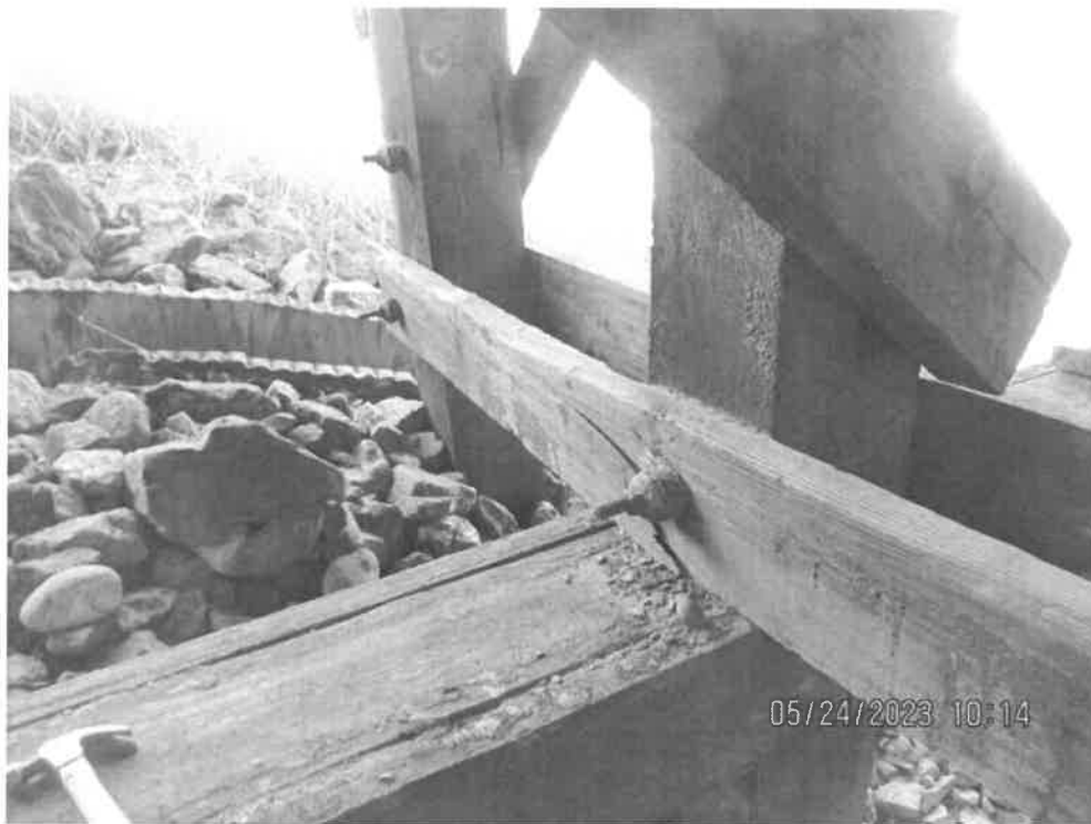
Photo 44: Broken timber brace (typ.).
