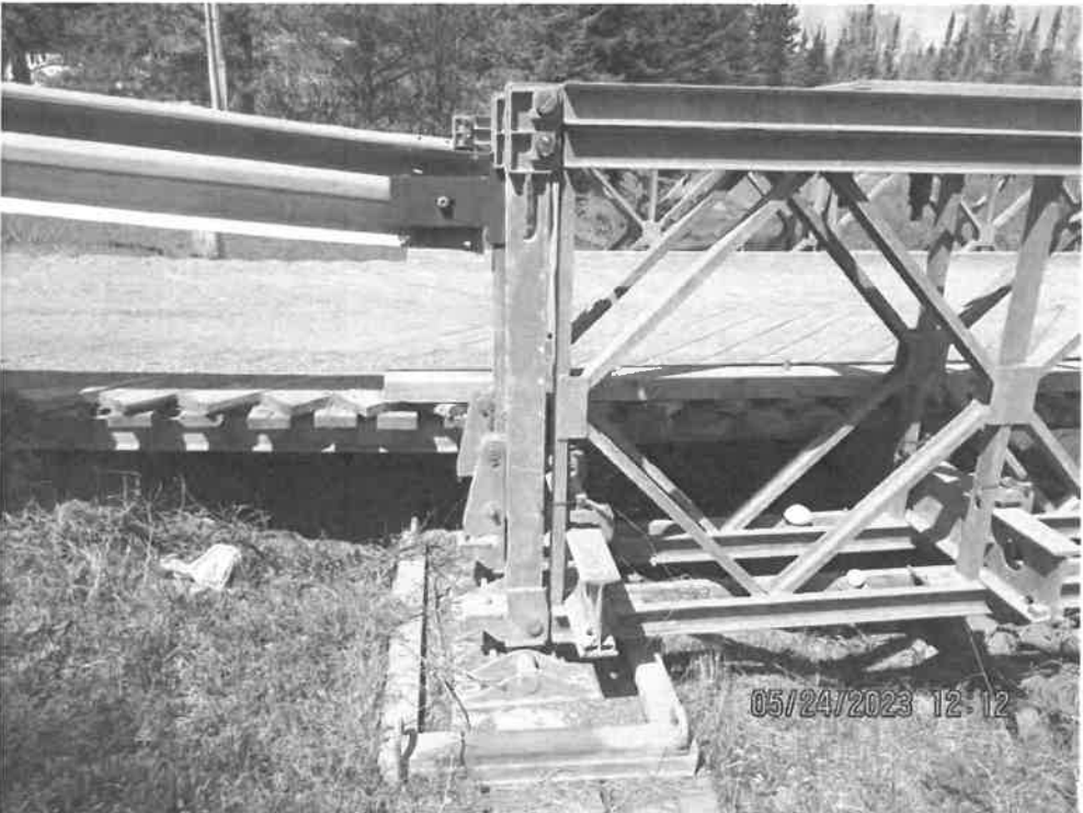
Photo 16: Improper connection of guide rail to bridge.
