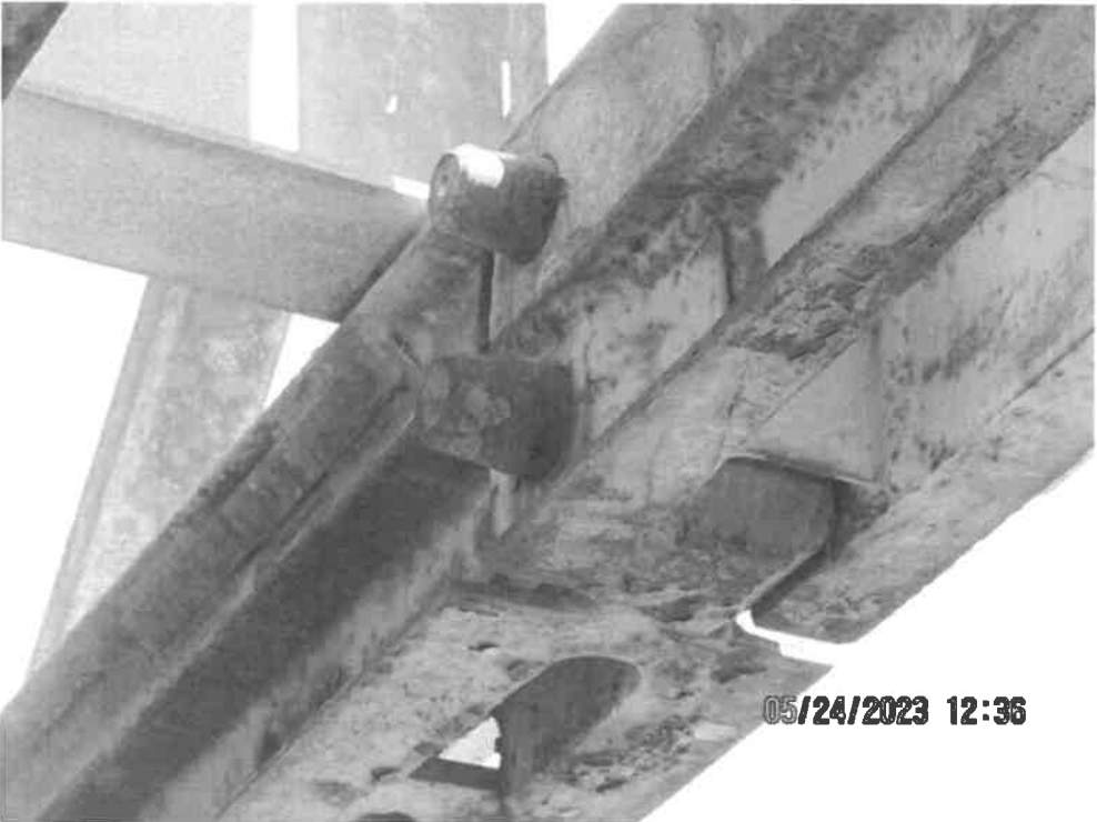
Photo 18: Loose cotter pin/panel pin.
