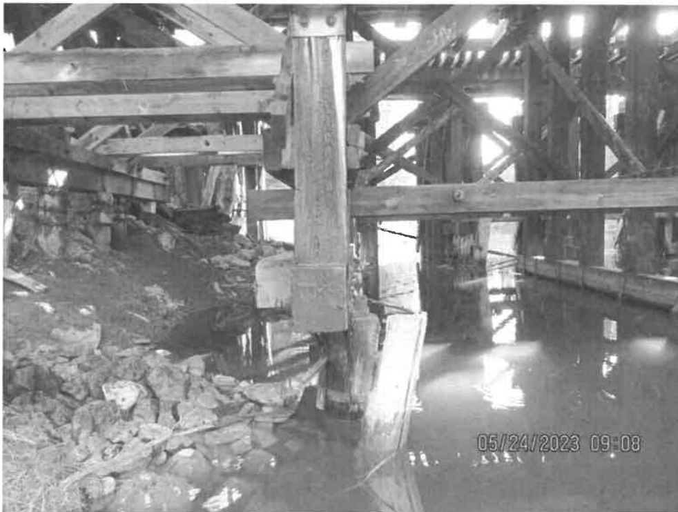
Photo 38: Pile not in full contact with pile cap (typ.).
