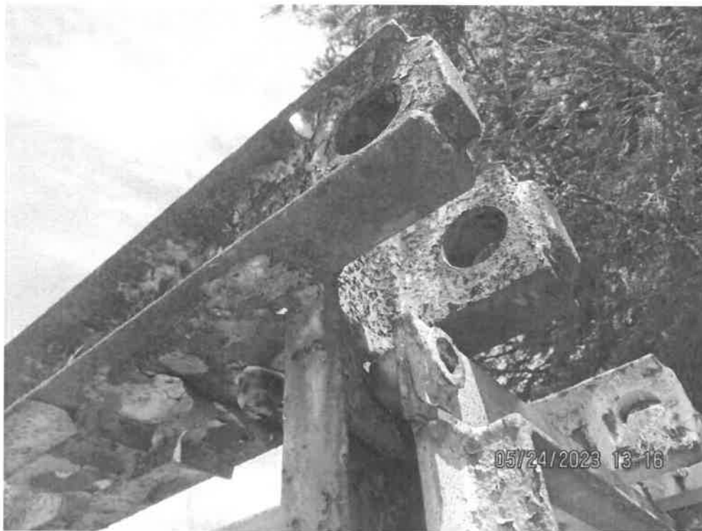
Photo 28: Missing truss brace bolt at southeast corner.
