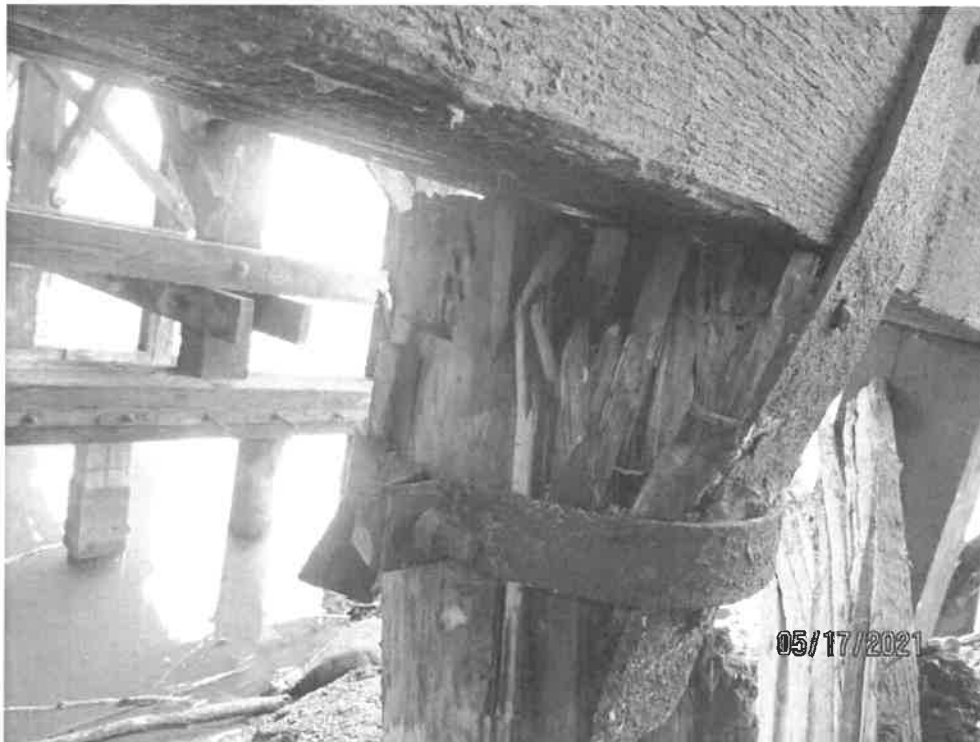
Photo 40: Severe rot and pile not in contact at Bent #12.
