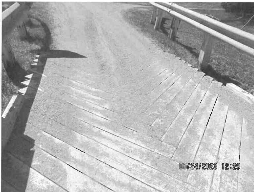
Photo 26: Gravel accumulation at approach ramp.
