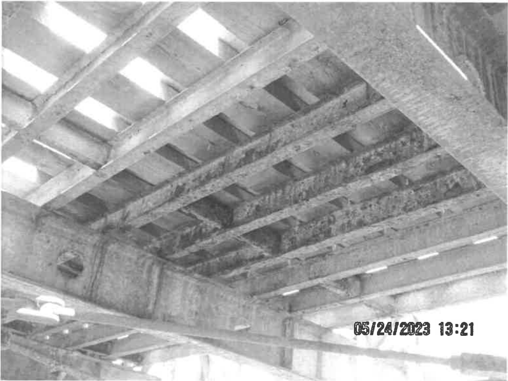
Photo 20: Severely corroded stringers (typ.).
