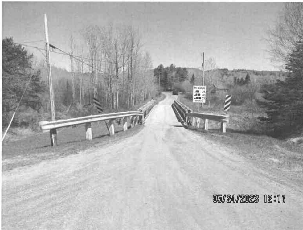
Photo 19: Guide rail mounted at improper height at southwest corner. Southwest Hazard Marker sign is leaning.
