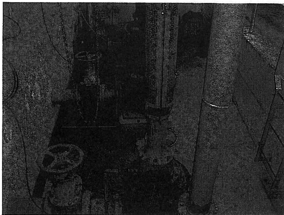
Photograph 8. Raw Sewage Pumps
